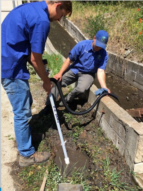
This leak was fixed at Kent Street (behind the Shell station)
