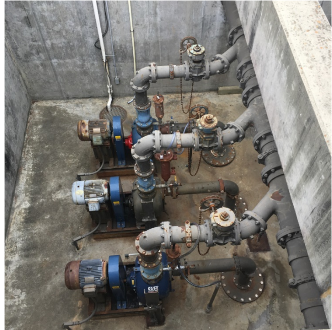
Figure 4: Influent pump station
