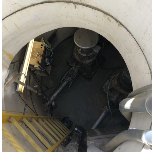
Figure 16: Lift station B4
