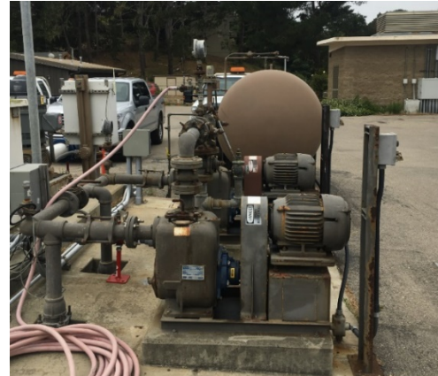
Figure 13: Secondary water pump station
