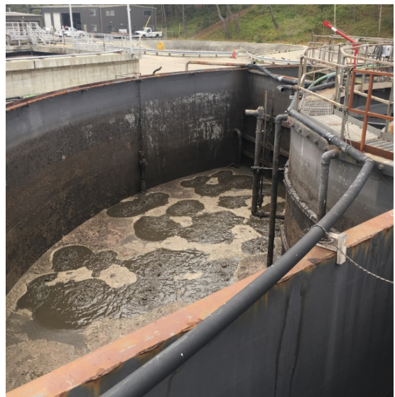
Figure 9: Sludge holding tank
