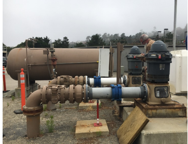
Figure 14: Effluent pump station
