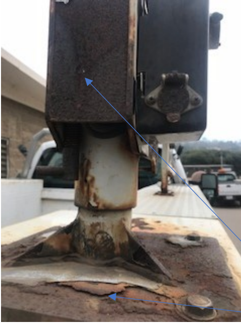
Figure 5 Lifting requirements have come off and the base is rusting
