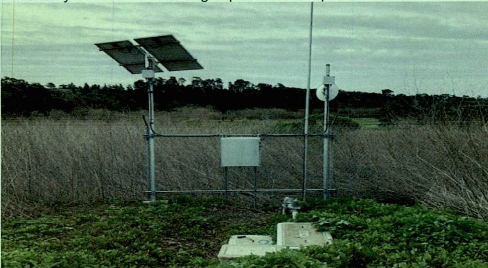
Relay Station at San Simeon Well Field
