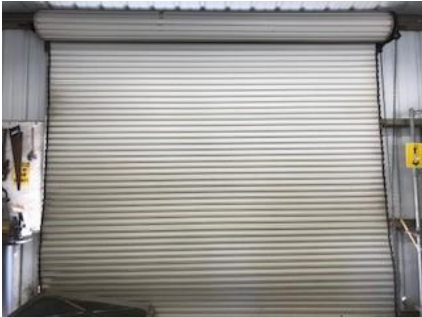
This is the 12'X 10' door after it fell.
