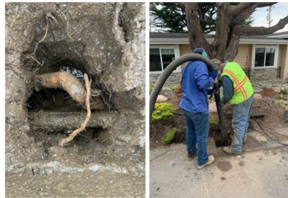
Figure D - Christmas Eve leak repair caused by root intrusion.
