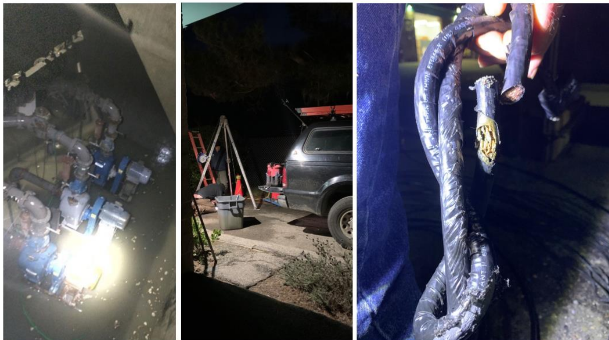
Figure 2 - Influent pump station flooding (left); late night repairs (middle); bad wiring (right)
