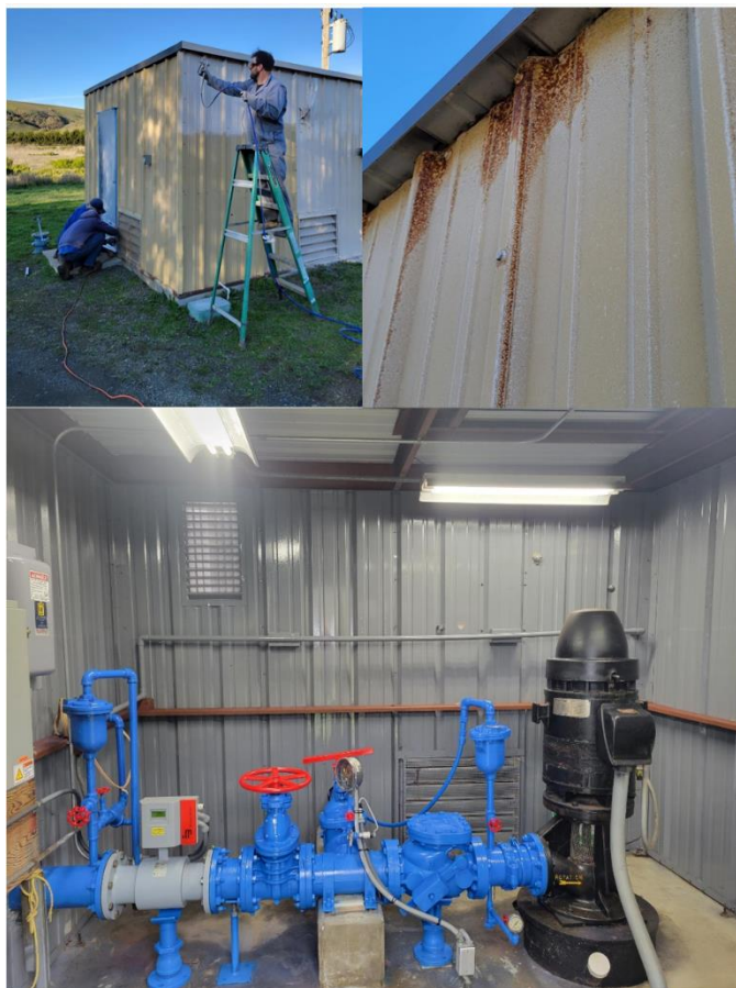
Figure 3 - Exterior coatings being applied (top left); rusting exterior before coating (top right); interior coatings (bottom)
