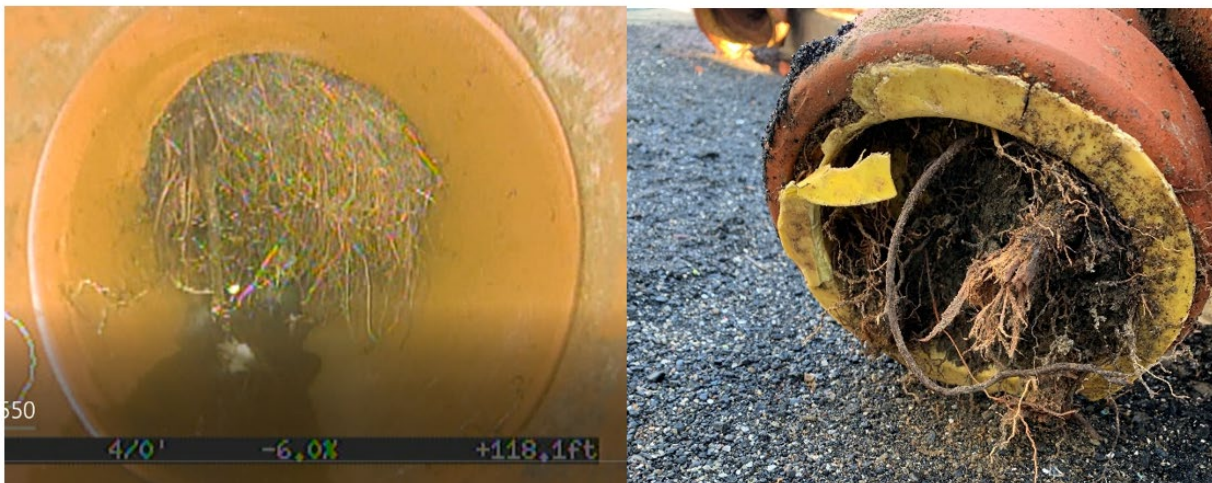
Figure D - Root intrusion viewed using the sewer camera (left) and after removal (right)
