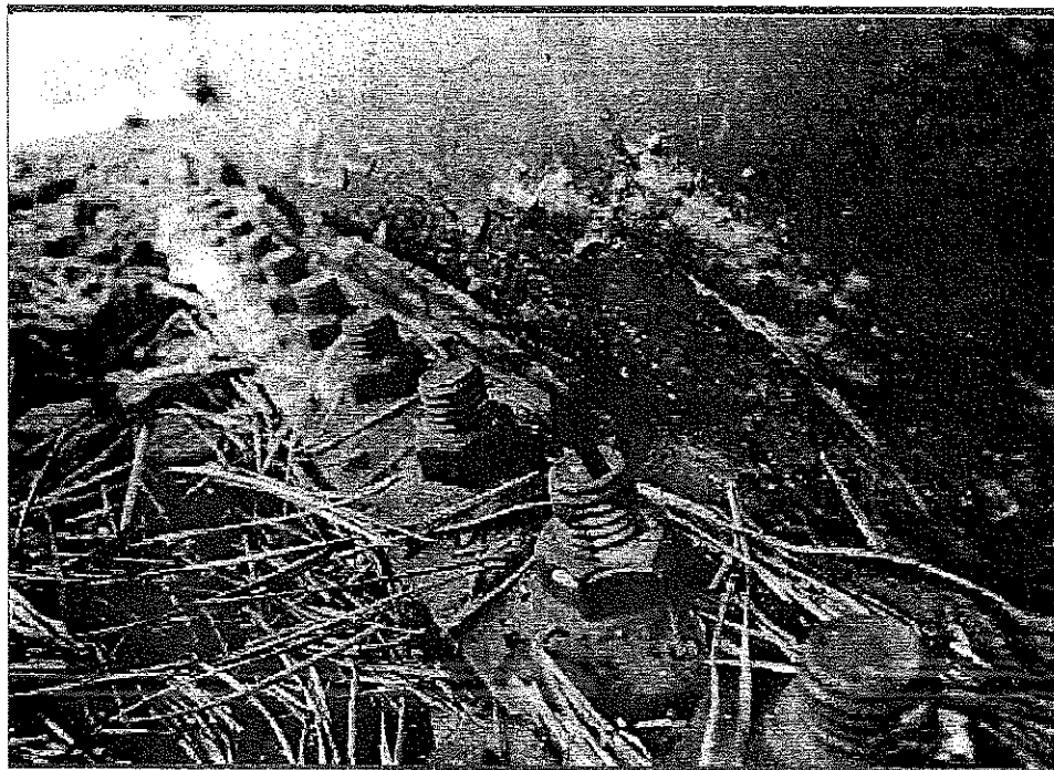
This is an additional view of significant corrosion and loss of structural material in the highly stressed lower shell.
