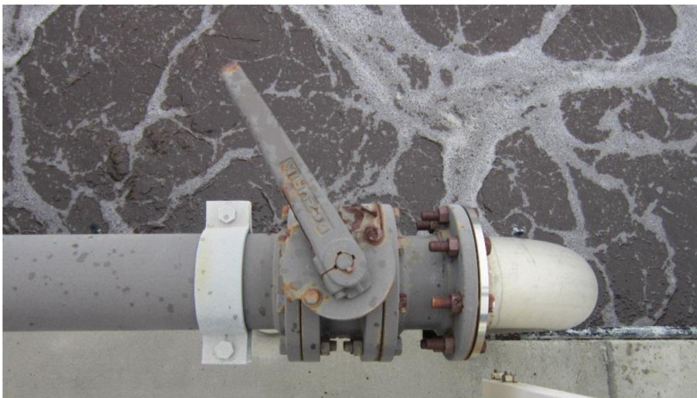
Figure 14: Partially Closed Blower Air Distribution Valve
