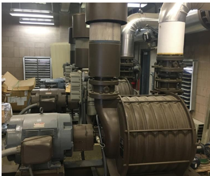
Figure 13: Existing Multi-stage blowers
