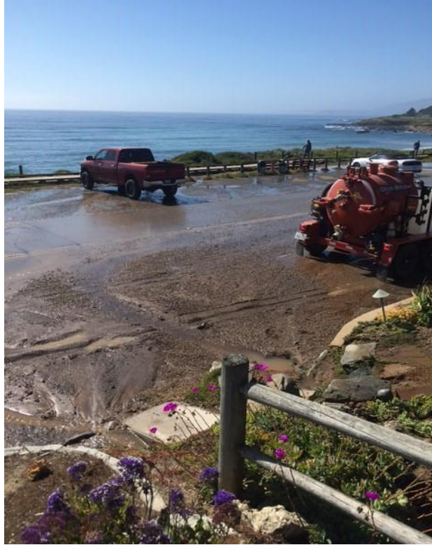
Moonstone Beach Drive leak on April 24, 2019
