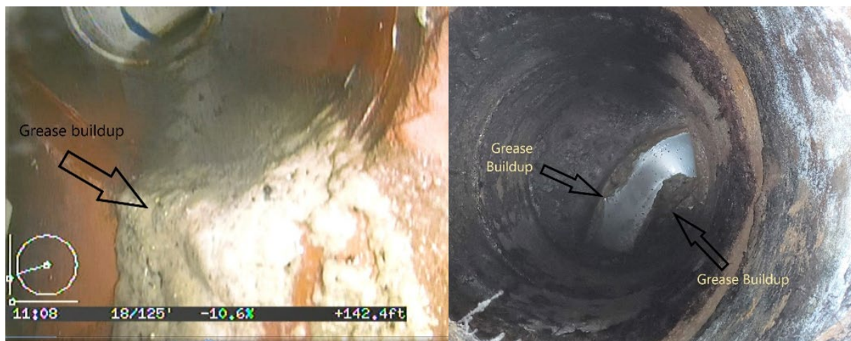
Figure C Examples of FOG buildup in the collection system
