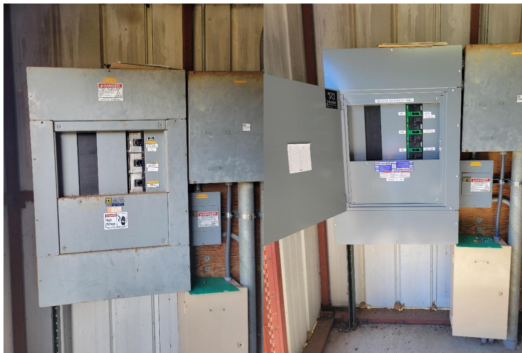
Figure F - Old (left) and new (right) electrical panel at the San Simeon Well Field
