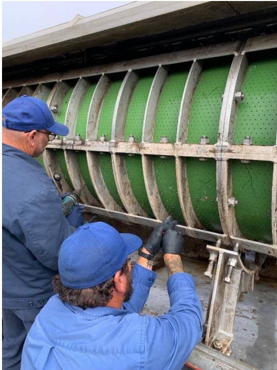
Figure A - Operators manually clean thousands of small holes in the screw press
