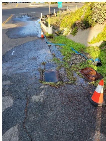
Figure C - Weymouth strikes again with new service line leaks this month
