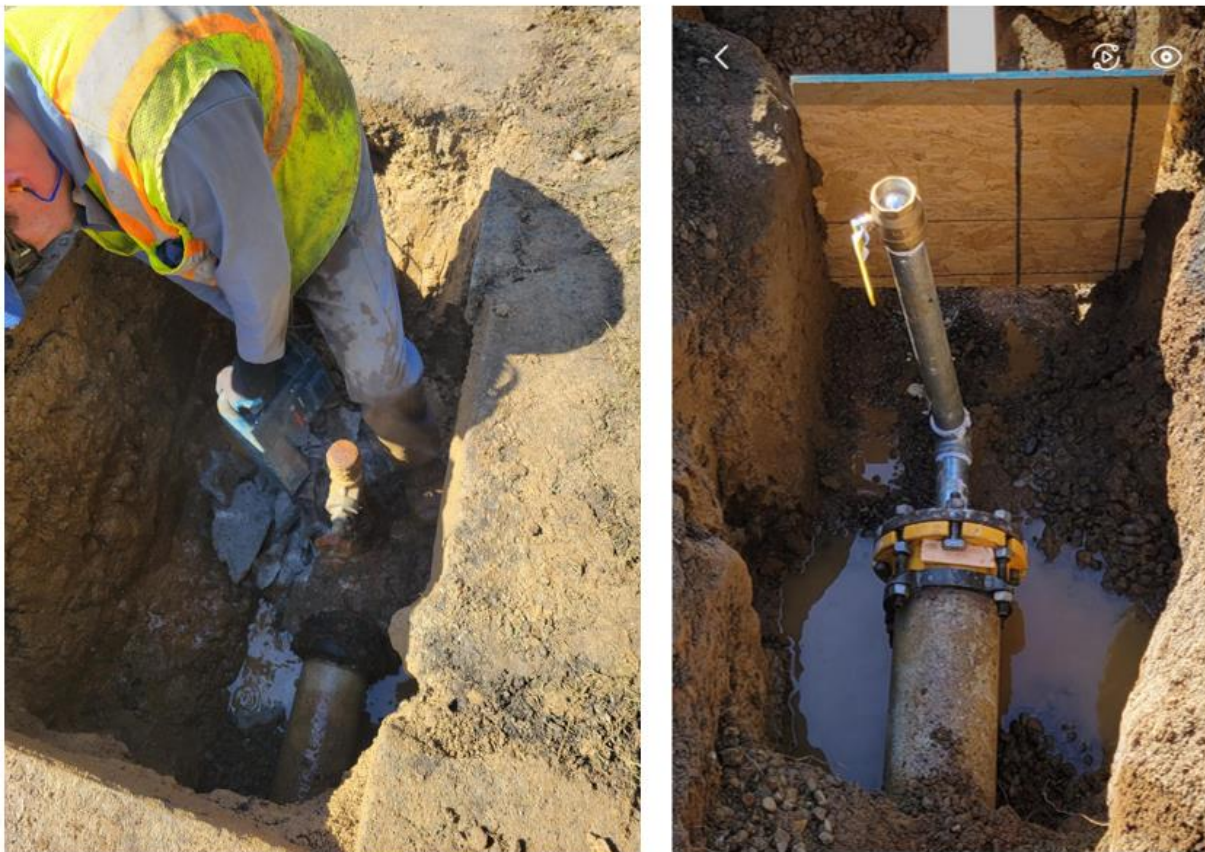
Figure E - Left: Water operator Art Garney removes by hand the thrust block at the dead end; Right: New dead end cap and blow-off are installed
