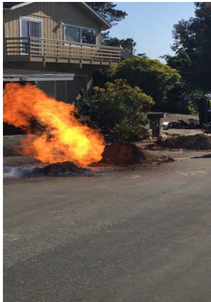
Figure 4 Underground SoCal Gas Company line catches fire. This illustrates the importance of marking underground lines before excavation.
