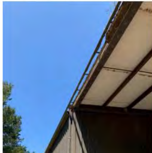
Figure 3 Maintenance is needed to extend the life of plant outbuildings.
