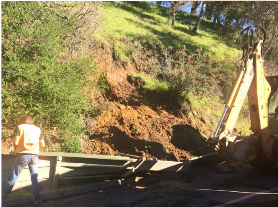
Minor Mudslide Behind the Ambulance Station on Main Street (January 2017)
