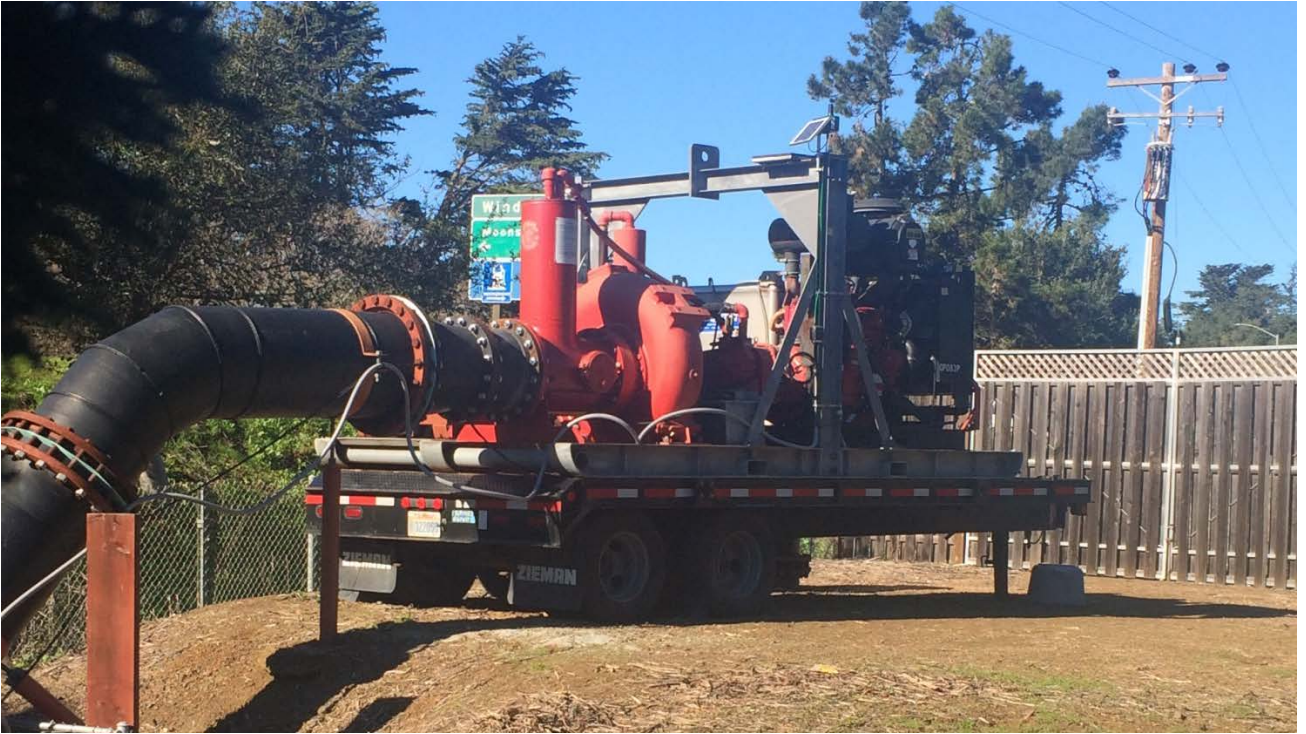
Flood Pump on Main Street - West Village
