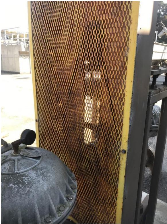
Figure 5 V belt at WWTP
