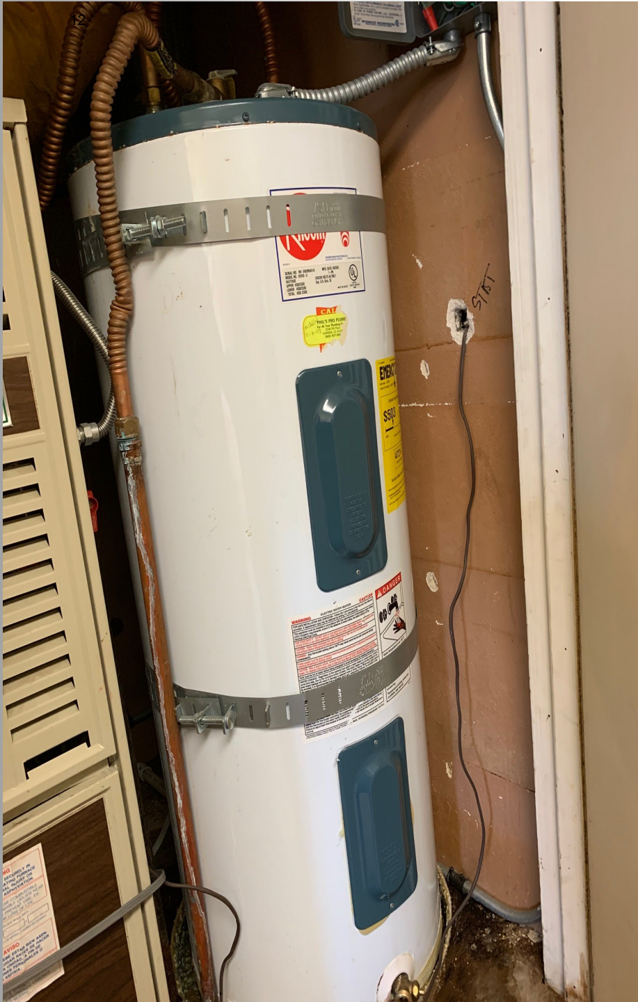
Old Water Heater for Kitchen
