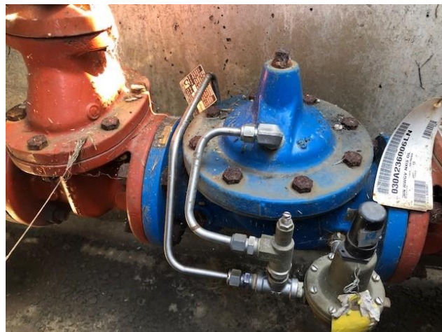
Figure 2 Six-inch Cla-Val pressure reducing valve in a vault on Madison Street.
