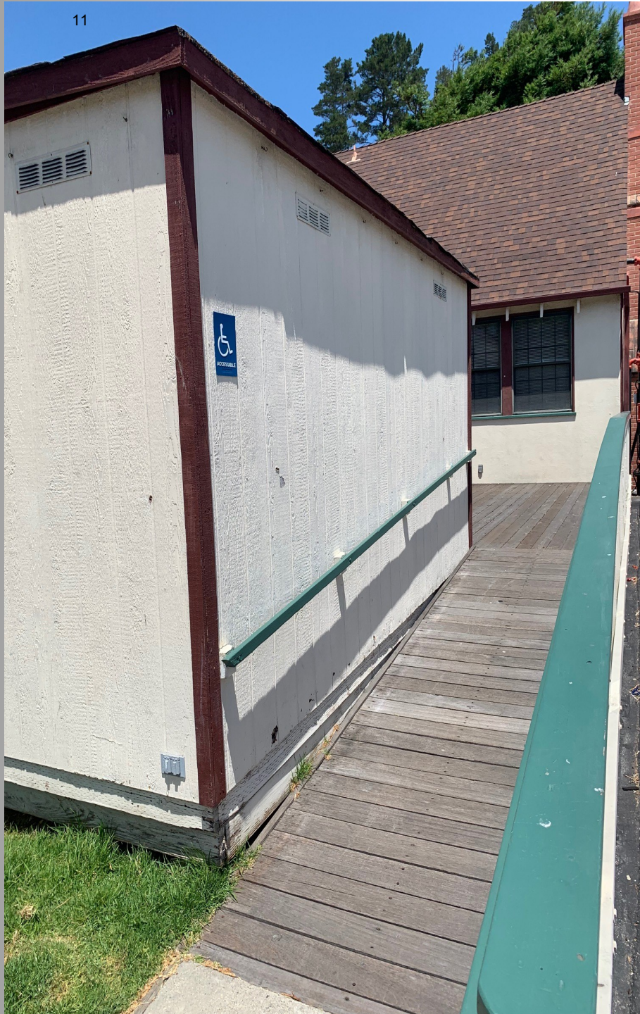
Old Leaky Roof, Rotted Siding and Fascia
