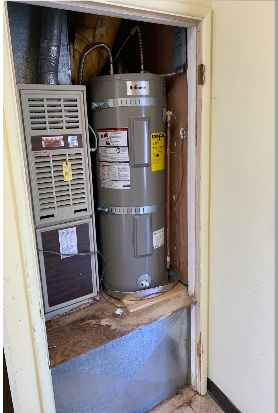
New Water Heater
