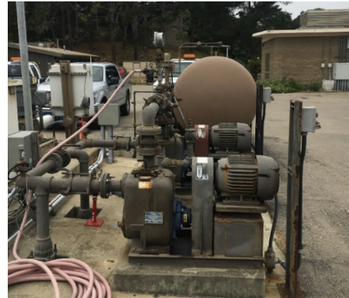
Figure 13: Secondary water pump station
