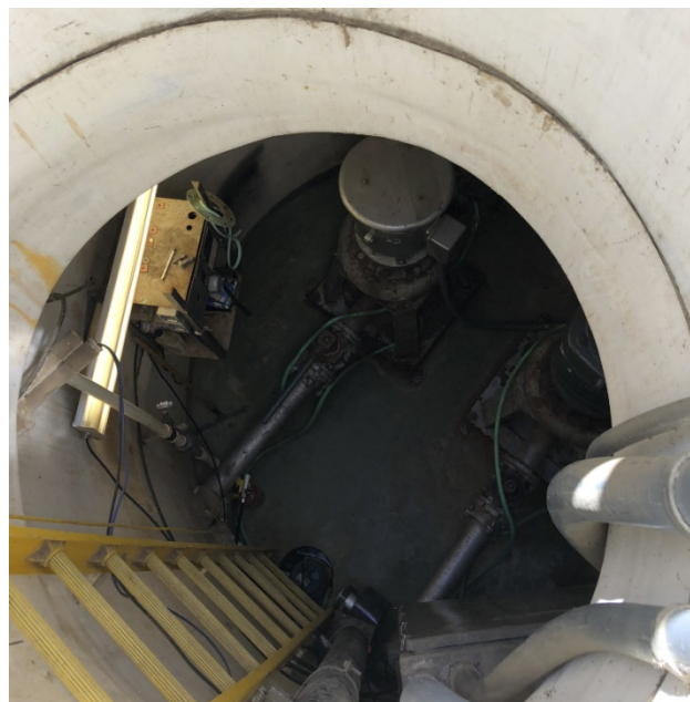
Figure 16: Lift station B4
