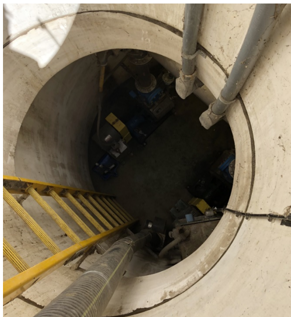
Figure 15: Lift station B1
