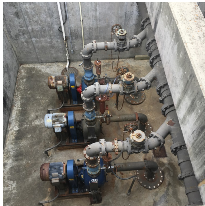
Figure 4: Influent pump station
