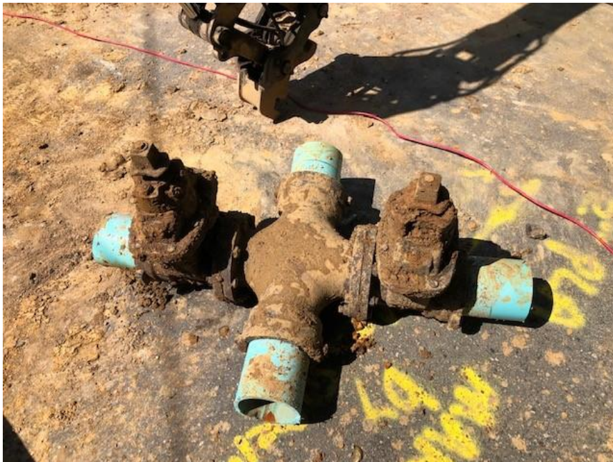
Figure 1 Original install of cross failure
