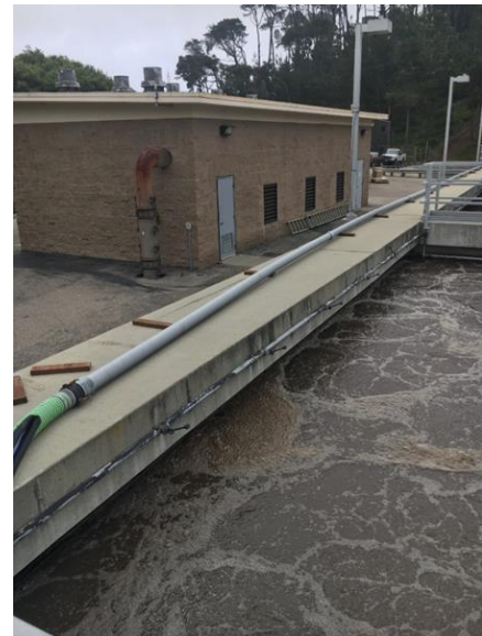
Figure 8: Aeration Basin and Blower Building
