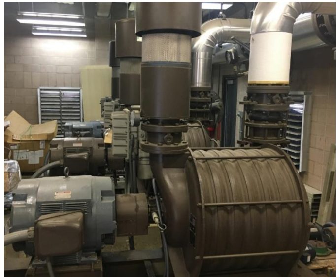
Figure 13: Existing Multi-stage blowers
