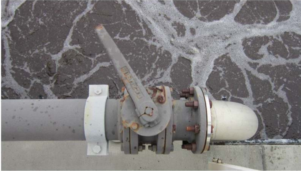
Figure 14: Partially Closed Blower Air Distribution Valve
