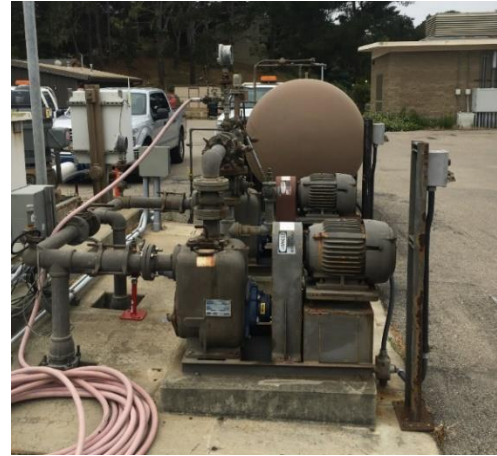
Figure 18: Secondary Water Pump Station
