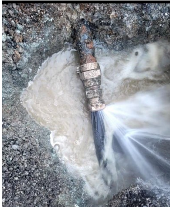
Figure C - A 2" steel line was the source of water loss in December
