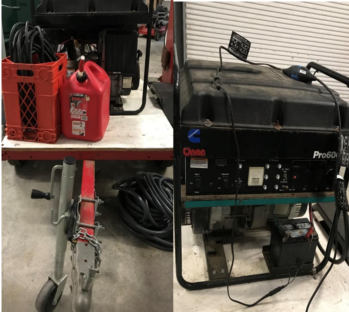
Generator for lift station 4 & 8
