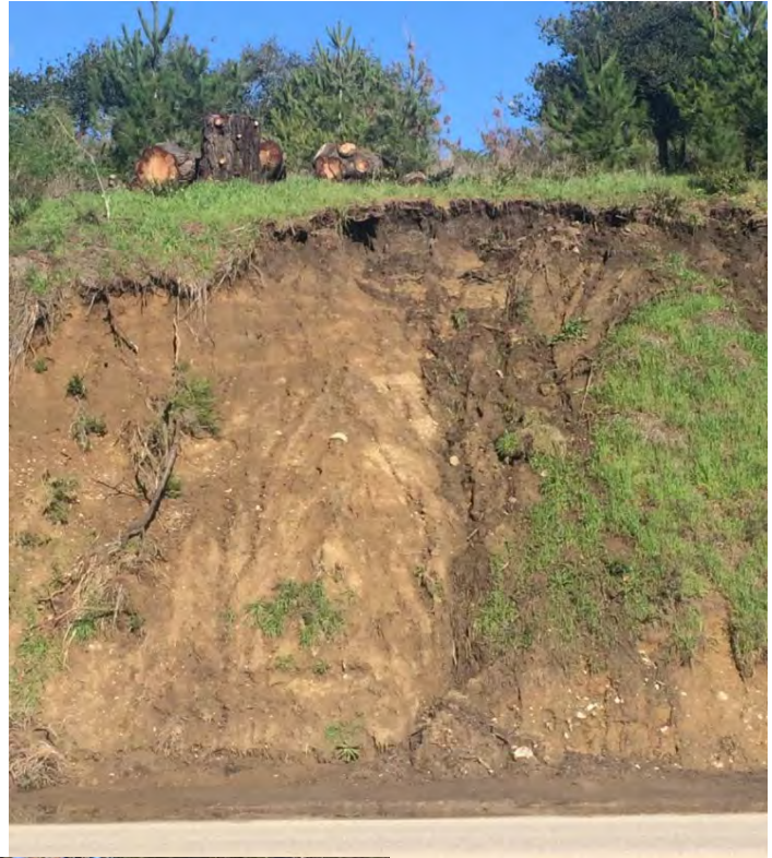
Minor Mudslide on Main Street Near Burton Drive (January 2017)
