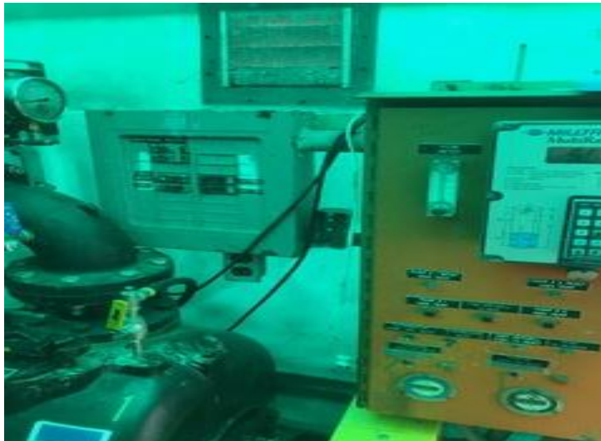
Figure 2: When completed this hydro ranger will be replaced with Opto 22 controls linked to the SCADA at the plant.
