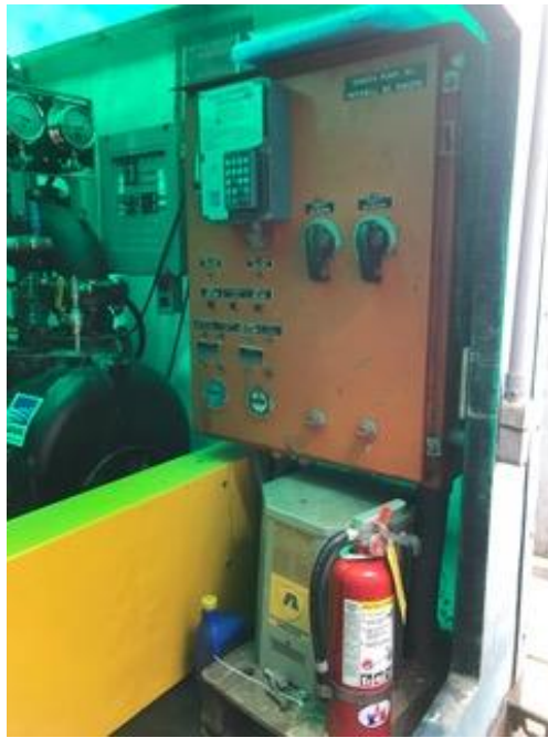
Figure 3: Here we have the electrical panel and controls.
