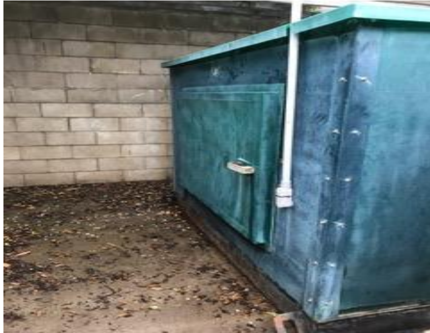
Figure 1: This is the housing for the pumps.
