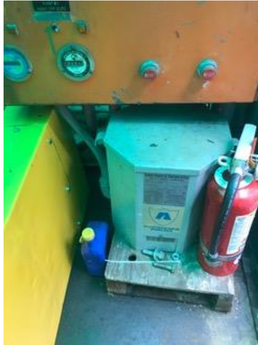
Figure 5: This transformer needs to be removed altogether, it can be replaced with one about 4 inches long added to the panel.
