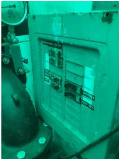
Figure 4: This is the uncovered breakers for the pump. Note its location to the piping.
