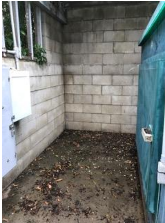
Figure 6: The proposal we place all of the electrical controls on this wall out from under the pump housing.
