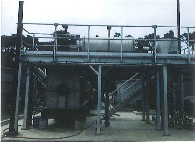
Figure 10: Sludge thickener and screw press
