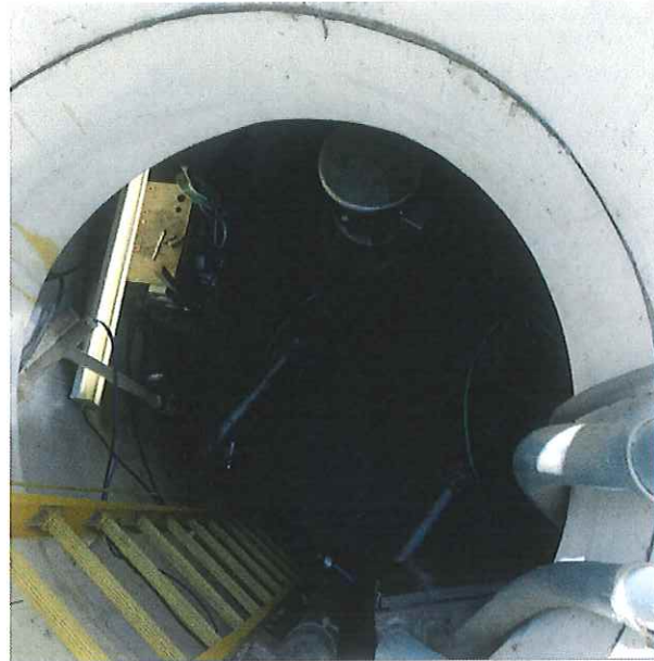
Figure 16: Lift station B4
