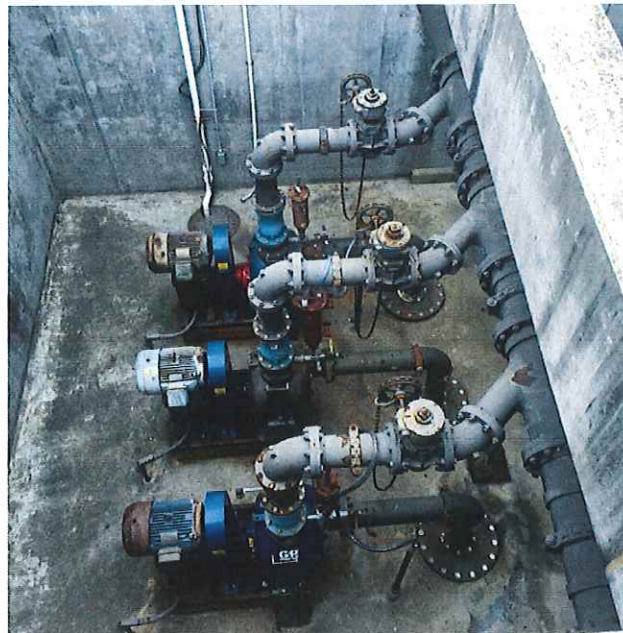
Figure 4: Influent pump station
