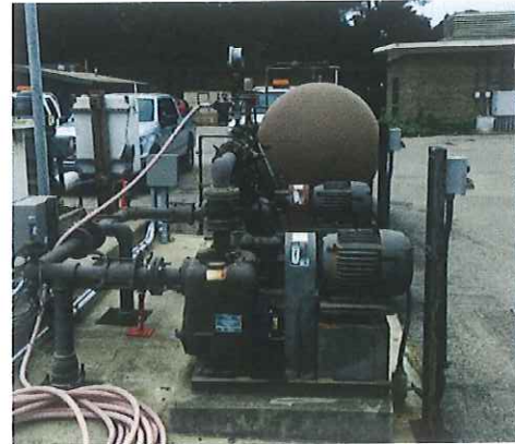
Figure 13: Secondary water pump station
