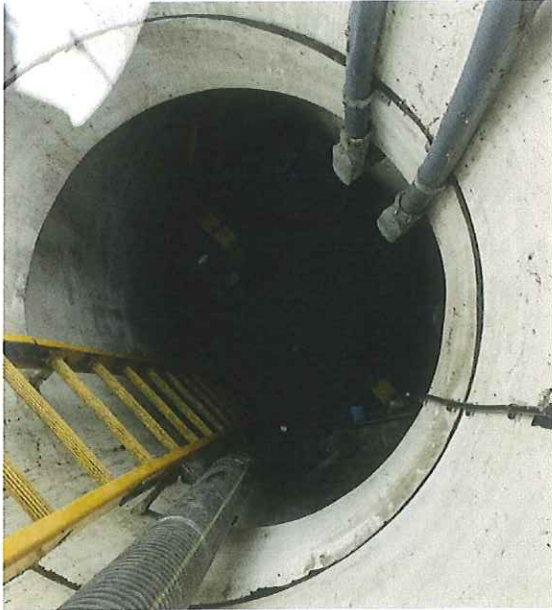
Figure 15: Lift station B1
