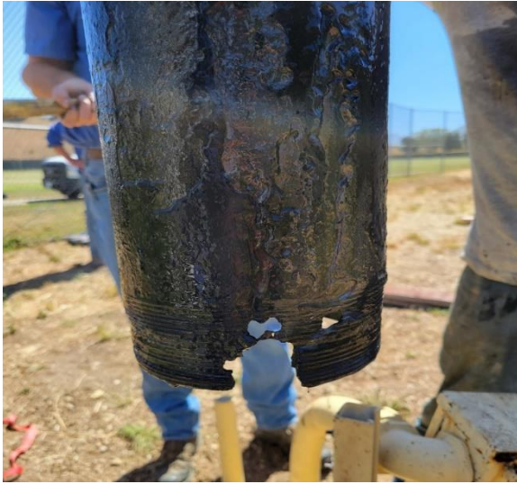
Figure A - SR4 well casing with corrosion at 81' below surface. This failure allowed silt to enter the suction pipe, contributing to failure of the pump impellers and motor and degraded water quality.
