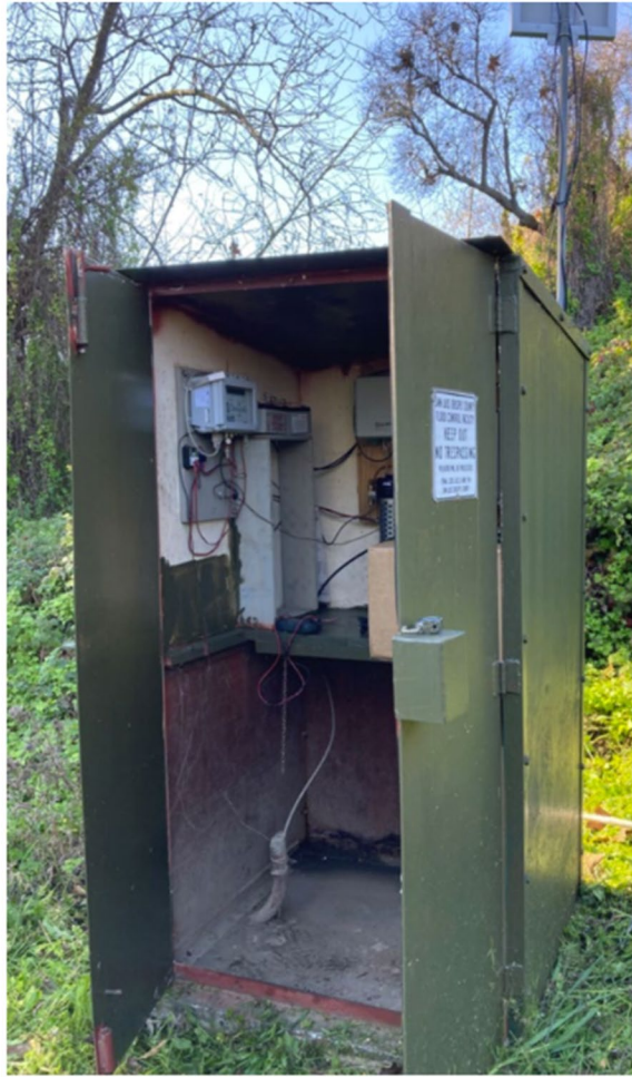
Photo: Lower San Simeon Stream Gauge Station structure - 3 ft x 4 ft X 6 ft metal housing on a portable concrete slab with 2-inch piping to the bottom of the creek.
