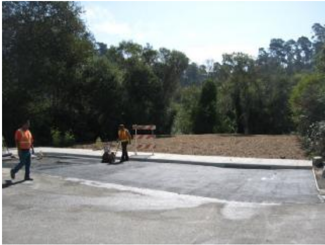
Bridge and Center Street Drop Inlet, New Sidewalk and Finished Lot with the County placing the Final Paving After 60-inch HDPE Culver Installation
