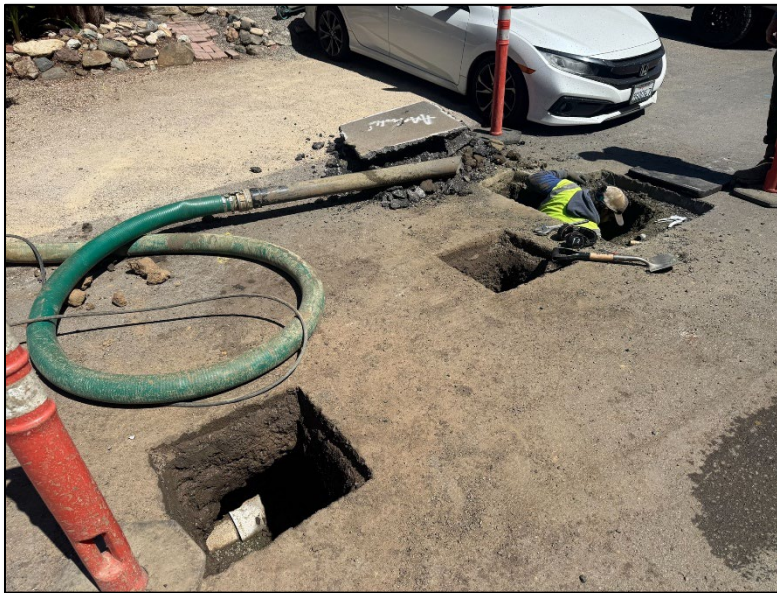
Figure 14: Potholing and excavation on Sheffield to locate leak
