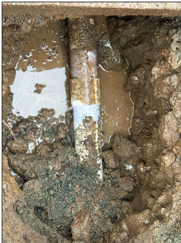
Figure 15: Leaking coupling excavated on Trenton
