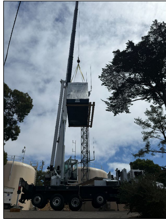
Figure 2: New generator lifting into position at Stuart Street
