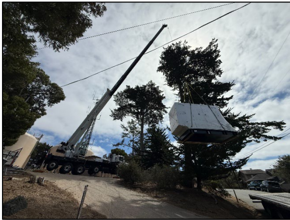
Figure 3: New generator lifting into position at Stuart Street
