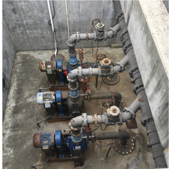
Figure 4: Influent pump station
