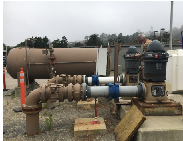
Figure 14: Effluent pump station
