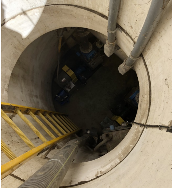
Figure 15: Lift station B1
