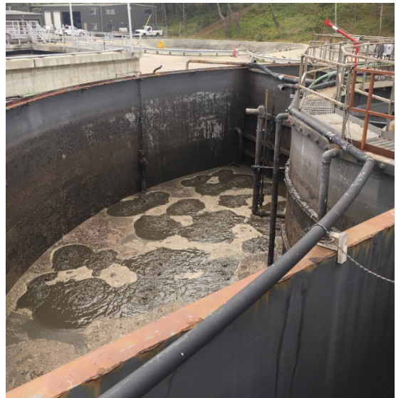
Figure 9: Sludge holding tank
