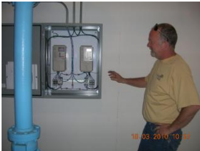
Jim Adams next to new Leimert Station VFD panel
