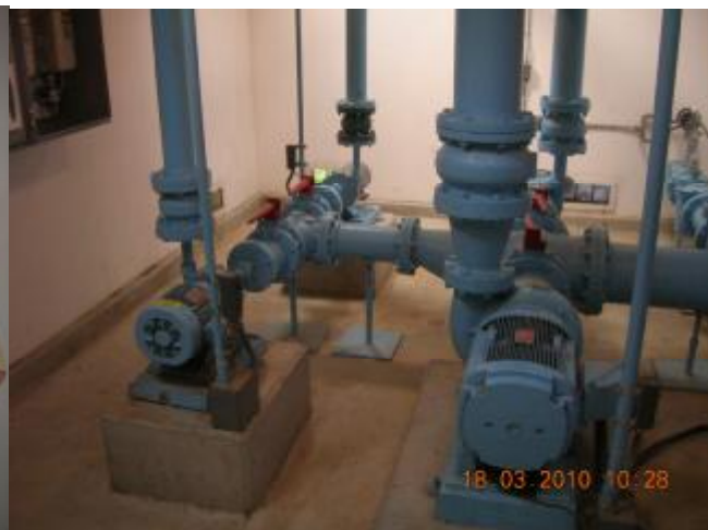
Pumps & Motors in the Leimert Station
